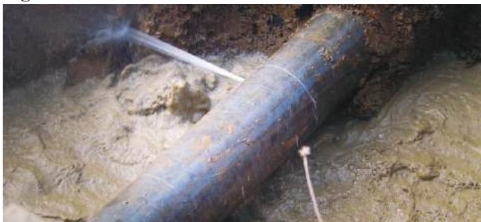
Figure 42. Confirmed water main leak.
