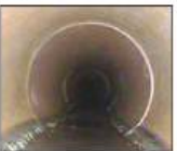
Vitrified Clay Pipe
