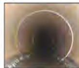
Vitrified Clay Pipe
