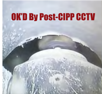
Damage to Lateral Not Present Pre-CIPP
