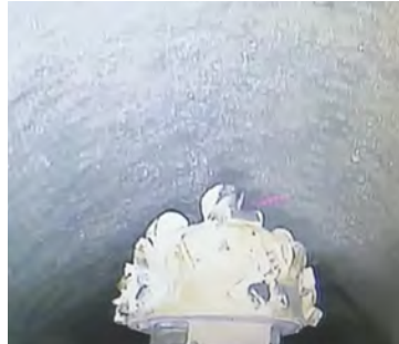
Poor Lateral Cutting Positioning
