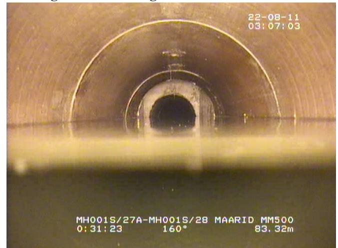
Figure 3. Surcharged ‘Inactive’ Sewer Main
