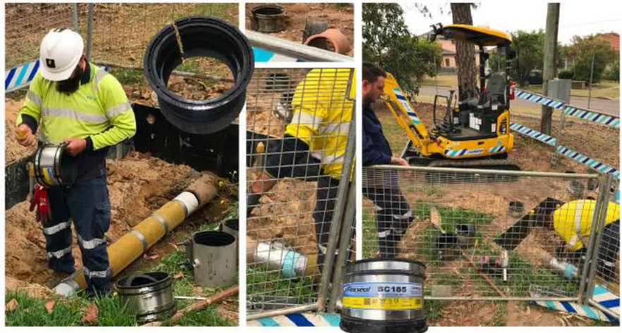
Sydney Water trial test bed for pipe evaluations.
