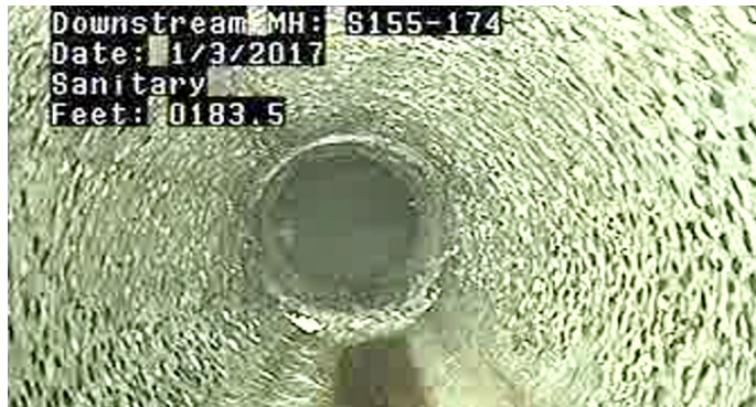
Figure 14: Example KCMO CIPP Pinholes
