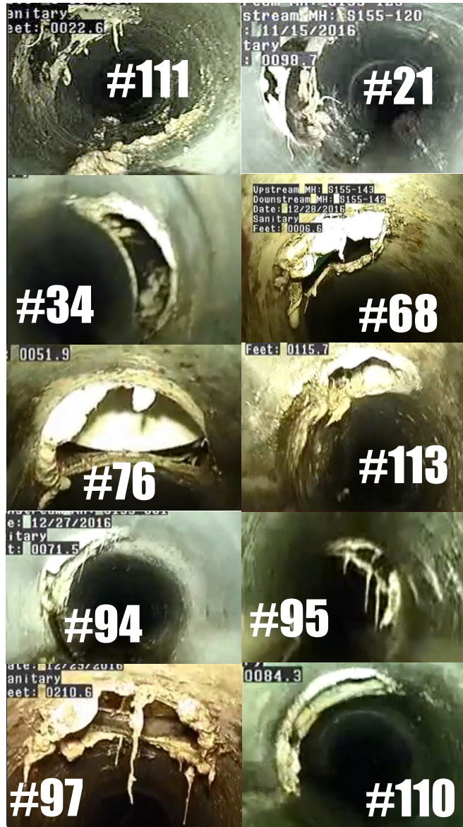
Figure 38: KCMO FELL Defects at PVC Connections
